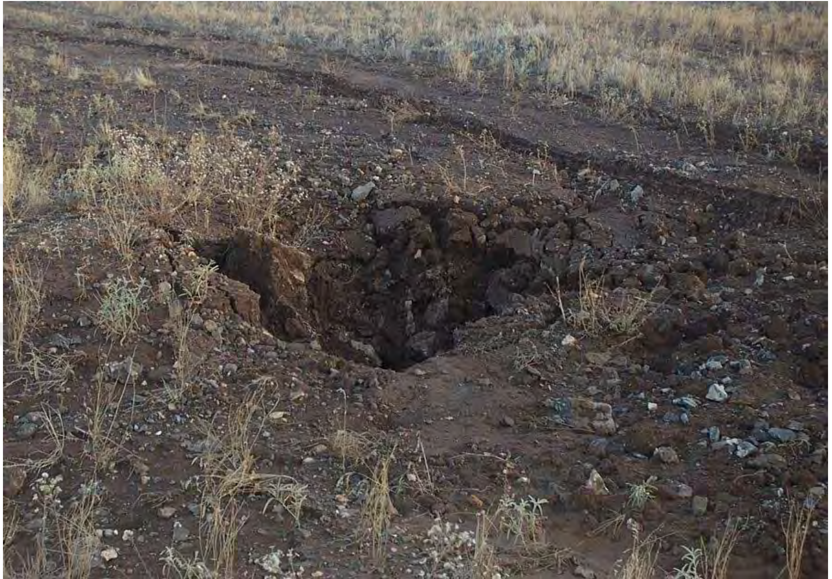
Failure During Hydro-Test
