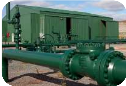
Compressor and Pump Station Noise
